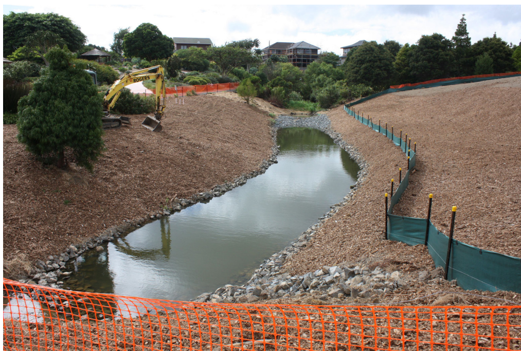
Fig. 7 Construction of a sediment forebay in 2010, with a channel dug into the streambed to capture stormwater from the neighbouring suburb before it flows into the ponds at ABG. Photo: Jack Hobbs.
