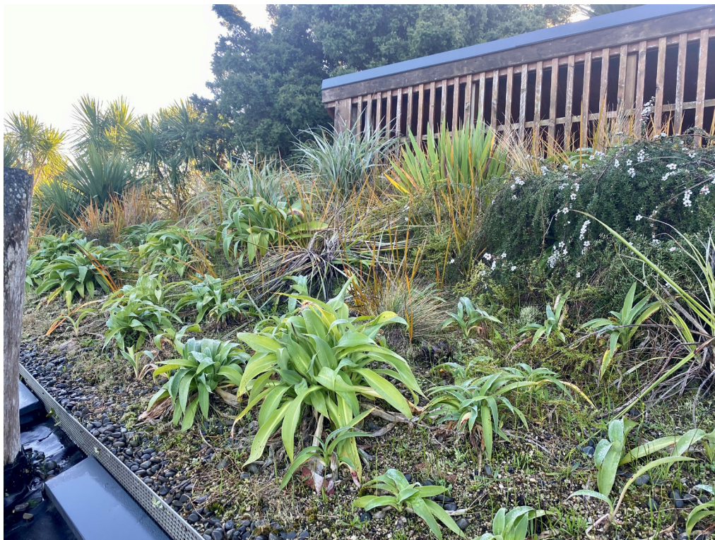
Fig. 9 Toilet block green roof planted with native species in July 2022. Photo: Emma Simpkins.
